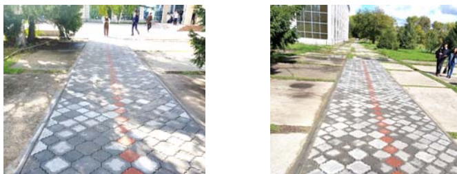
Figure 4: An experimental track laid out of paving slabs made at the experimental site
