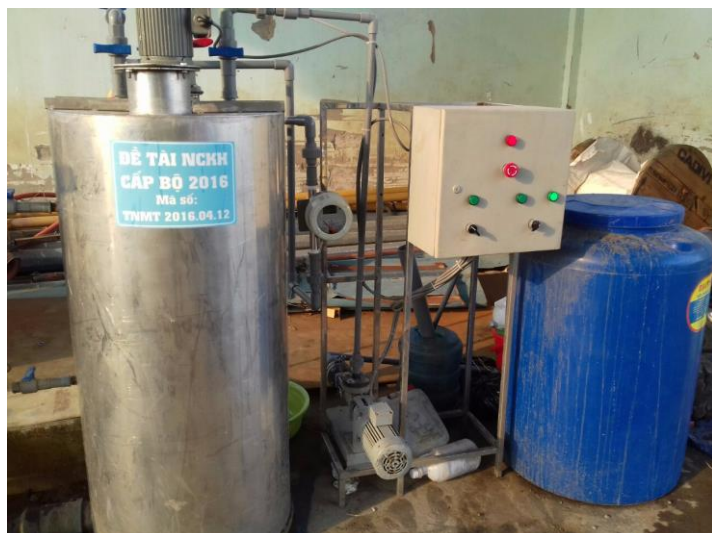
Figure 1: Anaerobic digestion reactor
