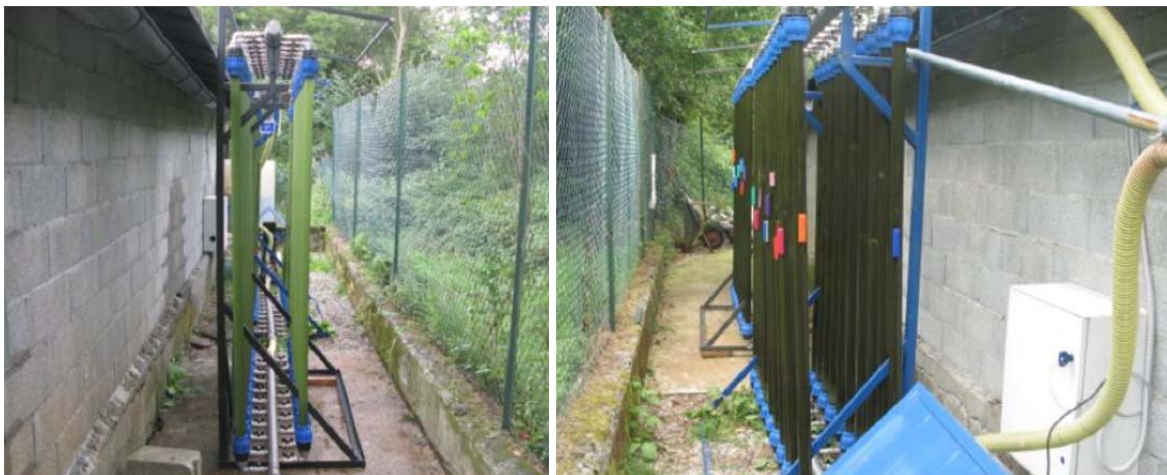
Figure 1a,b: Semipilot plant photobioreactor installed at San Pietro Vara (La Spezia, Italy) wastewater treatment plant.
