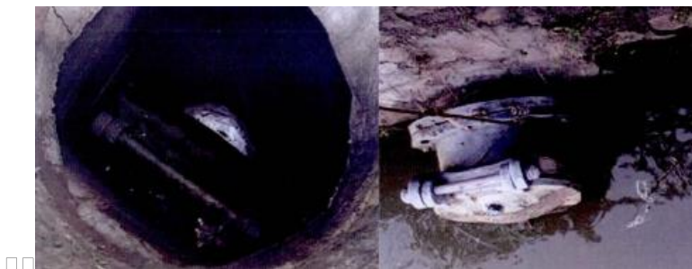
Figure 2: Cracks in the internal mouth and external mouth of the well□□
