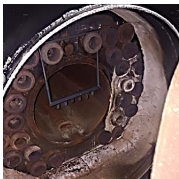
Figure 1: Back opening of the boiler, there the support of the samples is observed; which was located in front of the flame zone
