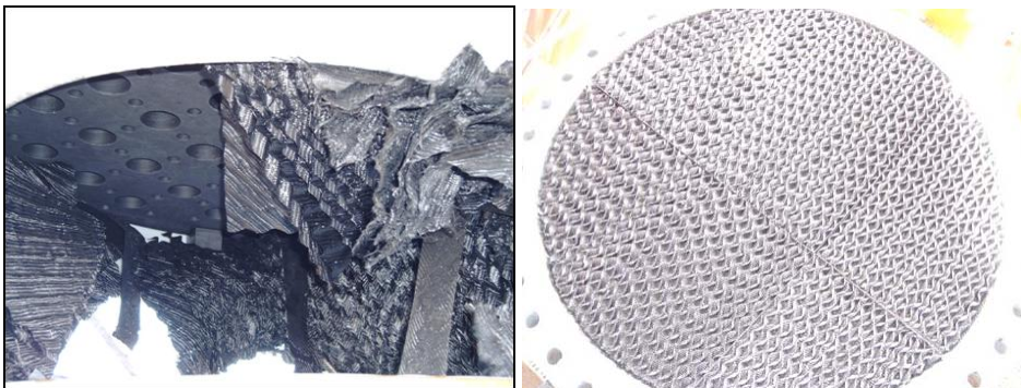
Figure 2: Left: Chimney tray made of graphite (view from below), with jammed Mellacarbon™ sheets; right: top layer of Mellacarbon™ of the upper section remained in place.
