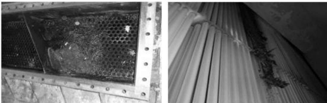
Figure 2: Fouling of the heat exchanger HE3 – tube side (left), shell side (right)
