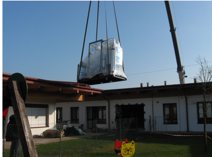
Figure 2. Installation of H 2 FC cogeneration system prototype
