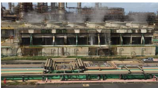
Figure 3: Cooling Tower studied from a Brazilian Refinery (Ávila et al., 2017)
