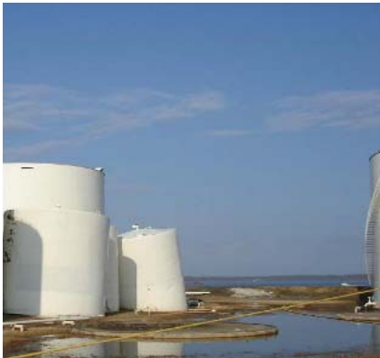
Figure 3: Overturning of a tank hit by hurricane Katrina, 2005 (LEF - Learning from Engineering Failures, 2012).
