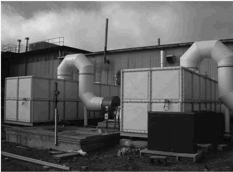
MÓNASHELL Enhanced Biofilter -First Commercial Application at B.P.I, Adeer, Scotland
