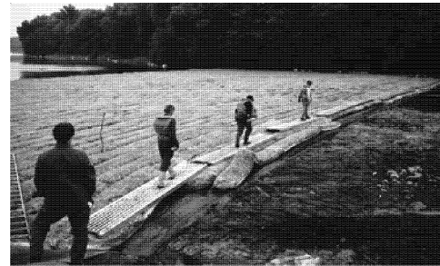
Fig. 5. Installing the biofilter of the extended area without boats from an already existing field
