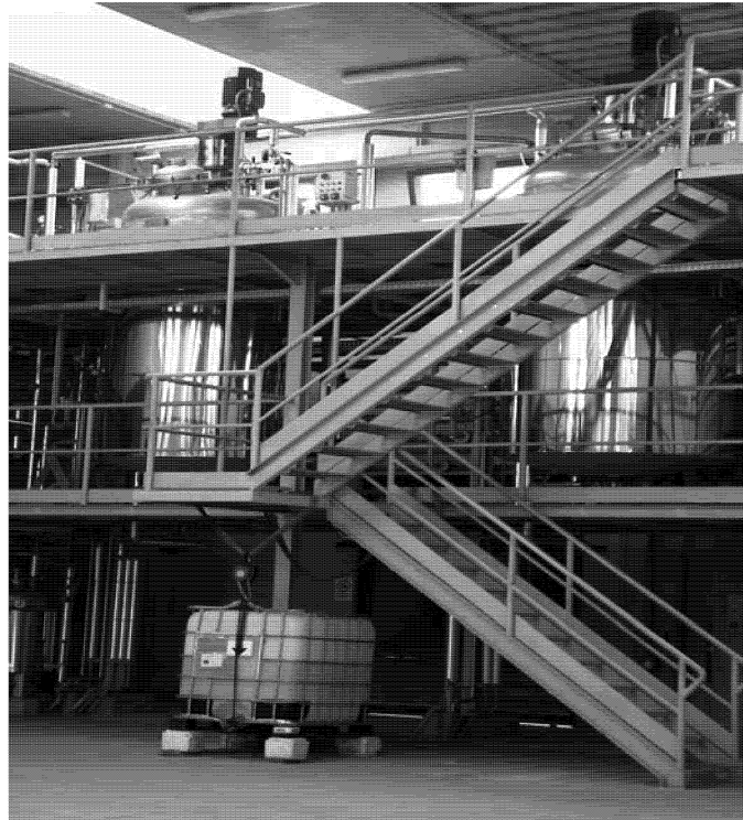
FIGURE 1 Bio & Geo Plant facility in Caserta
