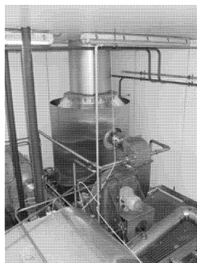
Figure 5 Equipment for the thermal treatment of off-gas from the smoked meat production
